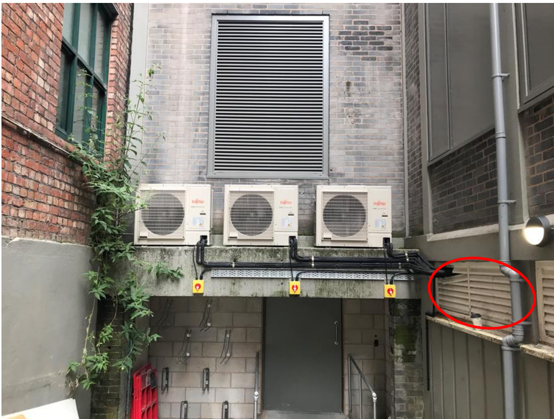
Figure 2 Photograph of installed plant items
