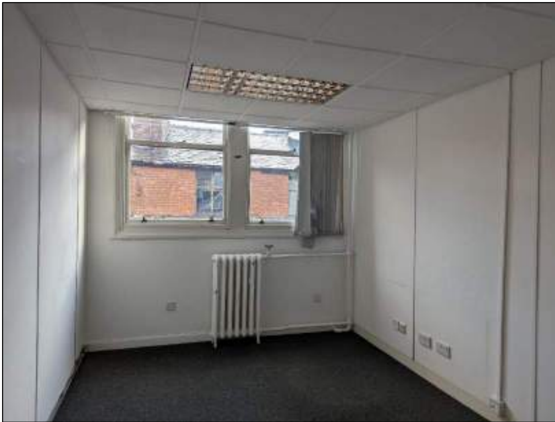
Plate 92: Small office with cast iron radiator
