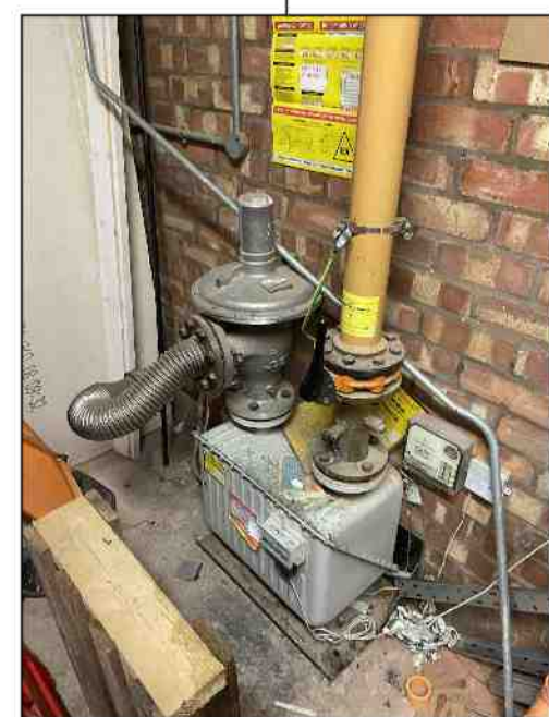
GAS METERS & ISOLATION POINT.
