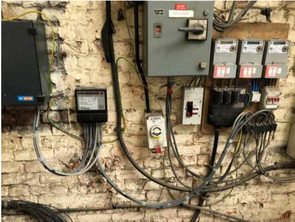
Photograph 13 Electricity supply to the main structure.
