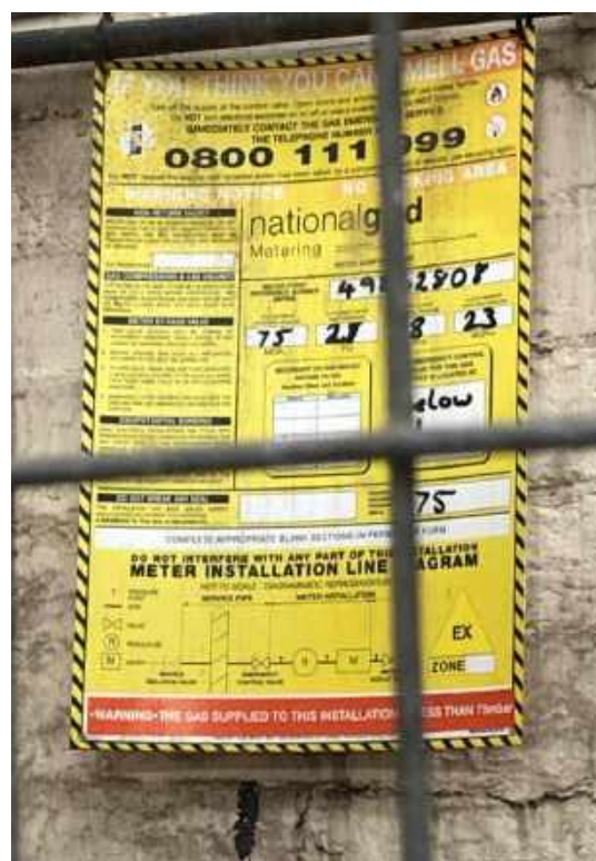
Photograph 12 Gas meter information.
