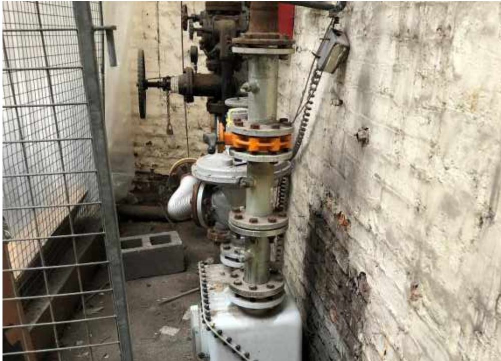
Photograph 10 Gas supply and meter to main structure.
