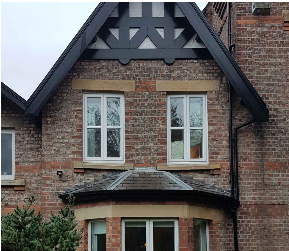
IMAGE 01: EXTERNAL ELEVATION ON STRUCTURAL OPENING TO BAY WINDOW. NOTE THE SIGNIFICANT DOWNWARD CRANK OF FIRST FLOOR WINDOW OPENINGS, DOWNWARD TRANSLATION OF CENTRAL PIER OF MASONRY
