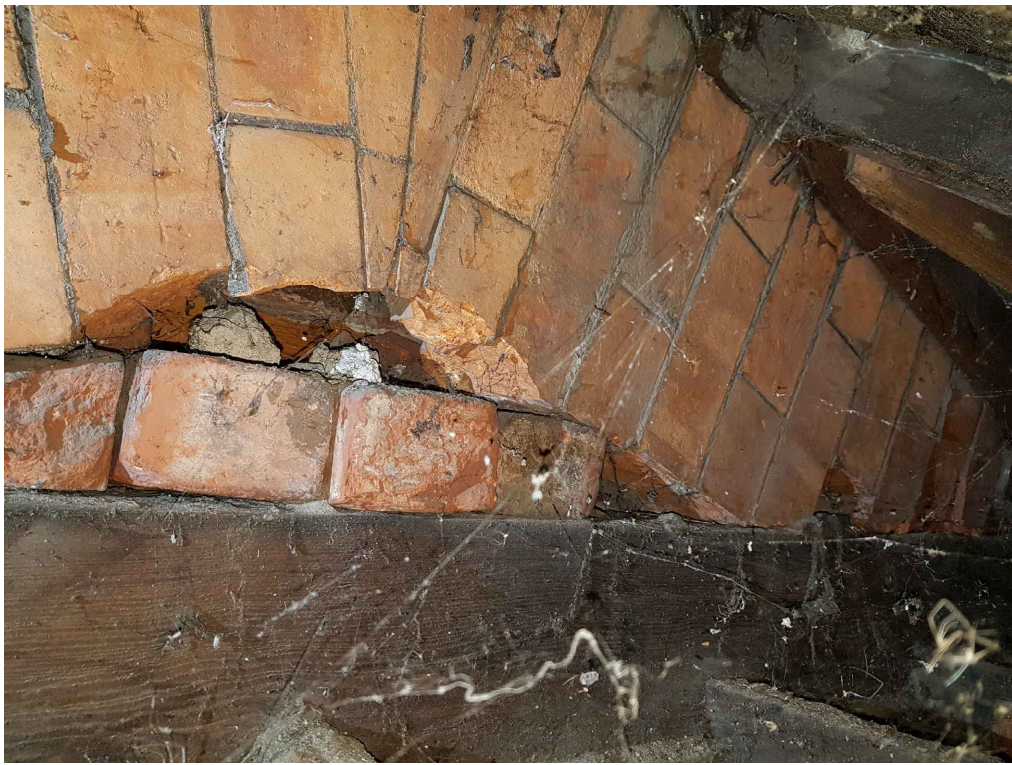
IMAGE 02: EXTERNAL VIEW OF RELIEVING ARCH OVER TIMBER BEAM SHOWING AWKWARD FLAT CHAMFER OF INTRADOS. DROP-OUT OF INTRADOS AND PACKING UNITS BELOW CROWN.
