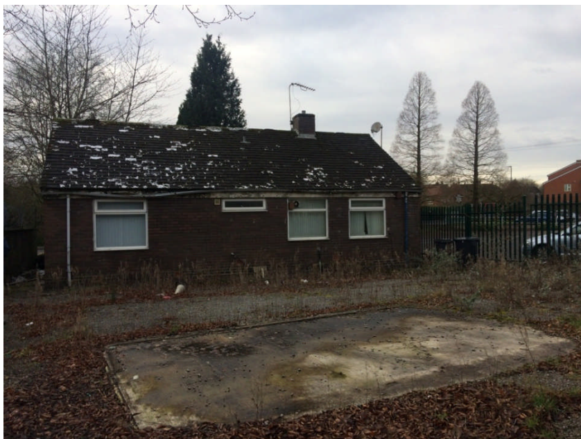
Photo 5: View south of northern elevation of bungalow (B2). Low bat roost potential created by gaps in timber boarding and roof structure caused by poor state of repair and water damage.
