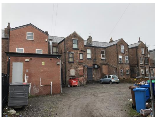
Extraction stack screened
