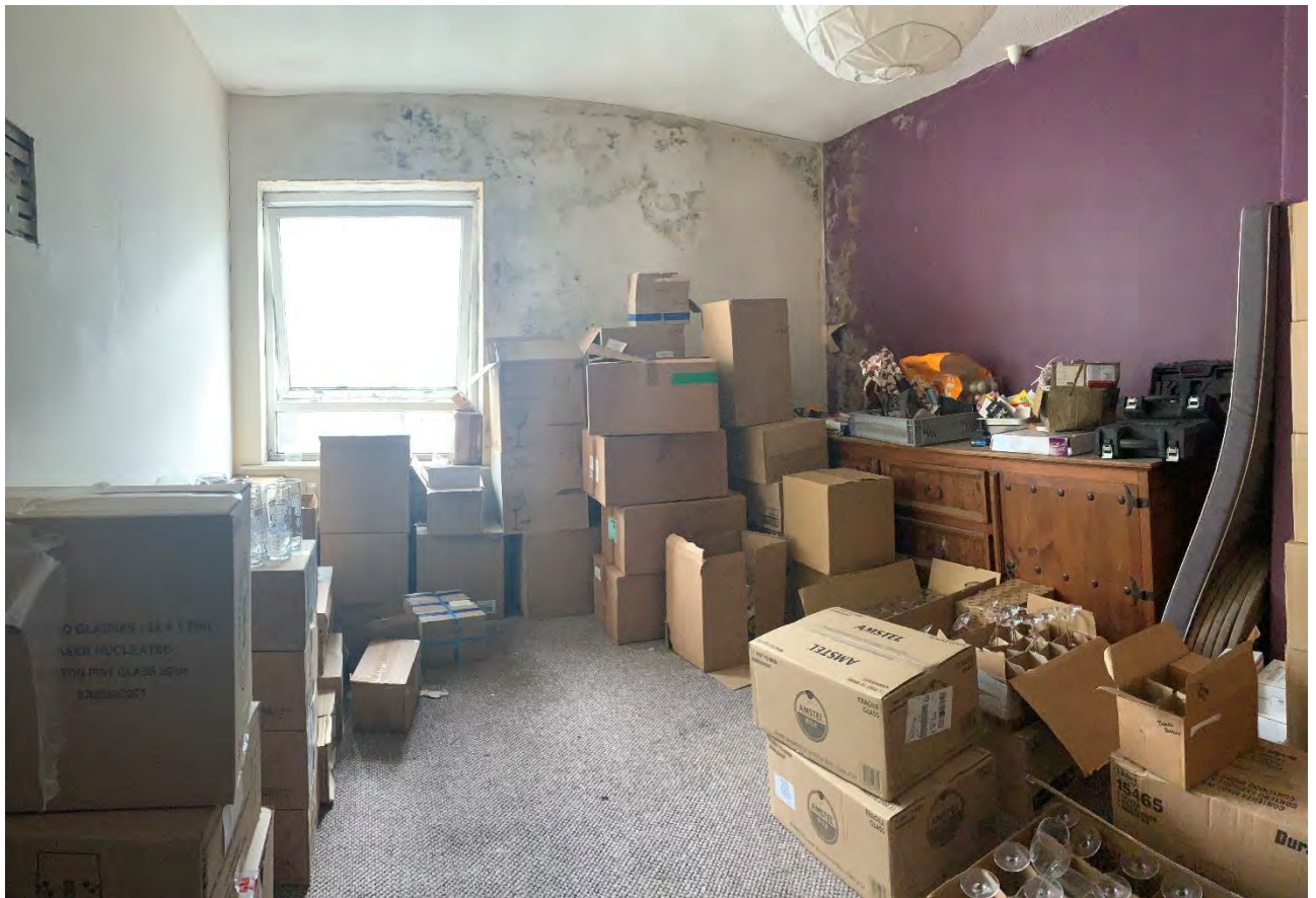
Image 4 - Photo taken 15th March 2022 during site visit, showing extensive damp to external wall.
