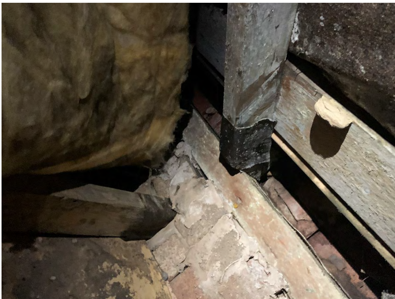
Image 5 - Photo taken 22nd March 2022 during site visit, showing floor joists into the base of the masonry parapet and rafters landing on top of the parapet. Timber ends are wrapped in plastic.
