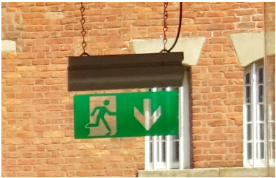
Existing fire escape illuminated signage
