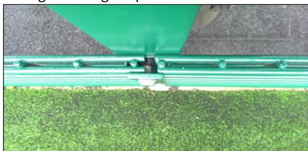
Figure 1: Image showing neoprene isolators
