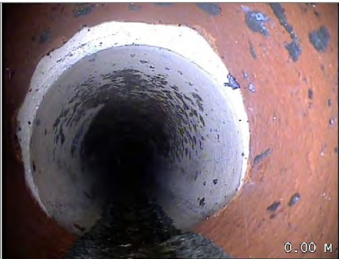
Start node type, manhole, reference MH 03
