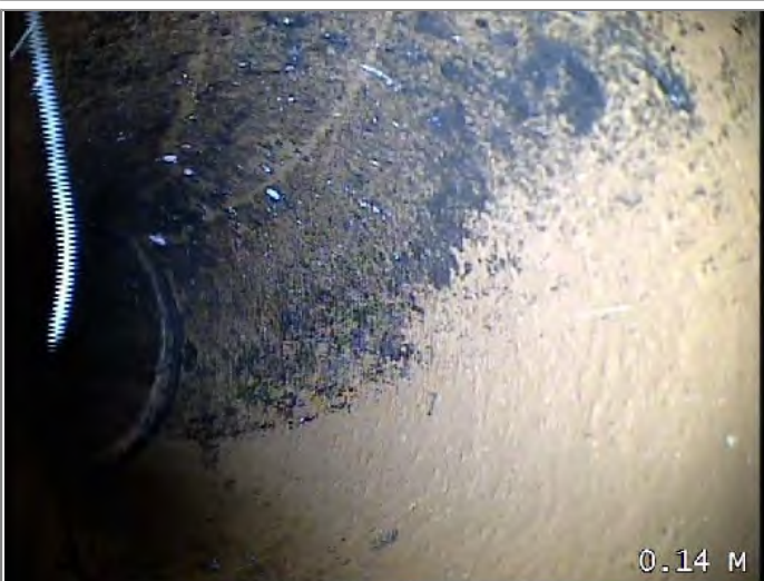
Line of drain/sewer deviates left
