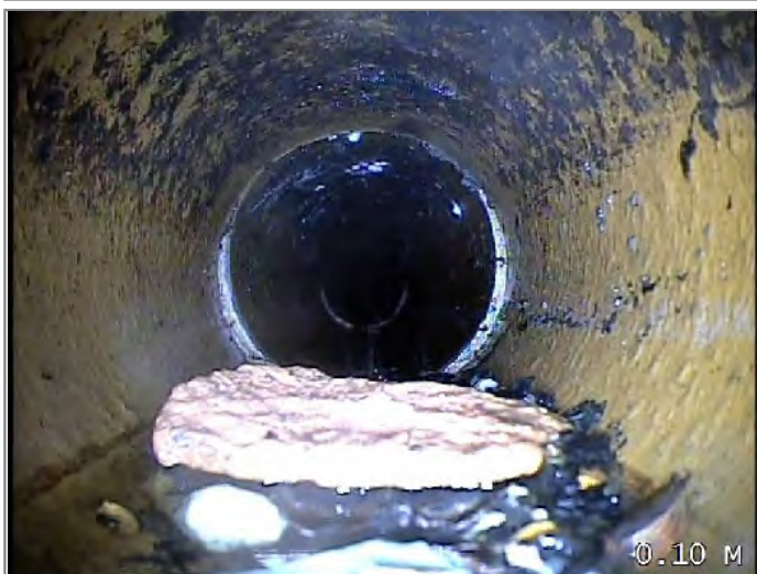
Settled deposits coarse 20% cross-sectional area loss
