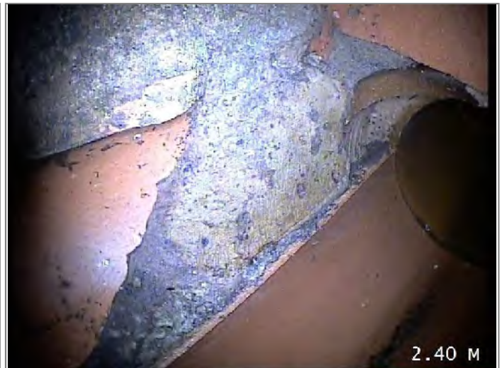
Finish node type, manhole, reference INTERNAL MH
