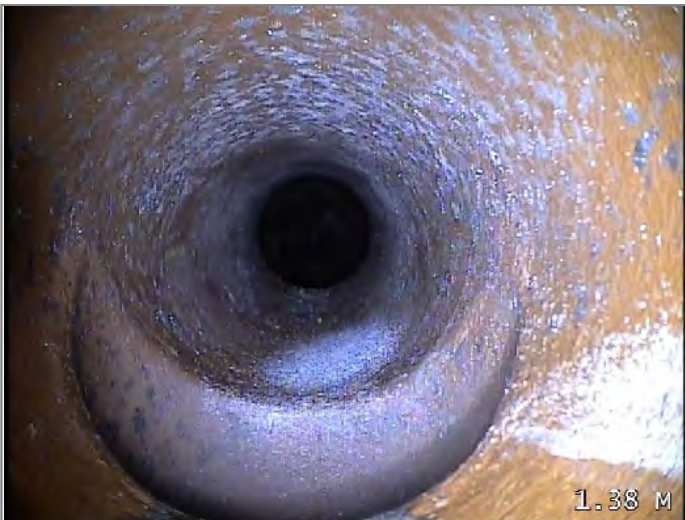
Line of drain/sewer deviates down - Remark: BACKDROP
