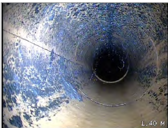
Crack circumferential from 2 to 9 o'clock
