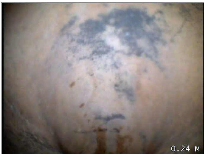
Line of drain/sewer deviates down
