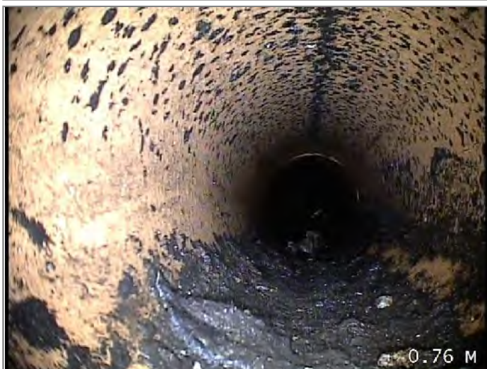
Settled deposits fine 10% cross-sectional area loss
