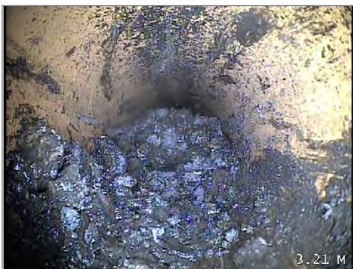
Survey abandoned - Remark: DEBRIS 75%
