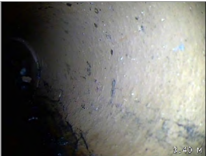
Line of drain/sewer deviates left
