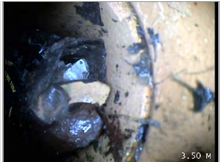
Survey abandoned - Remark: DEBRIS - 80%
