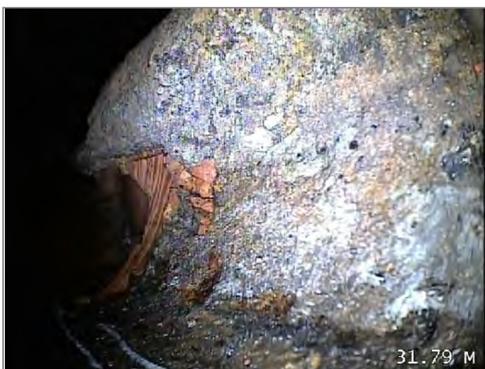
Finish node type, manhole, reference MH 03
