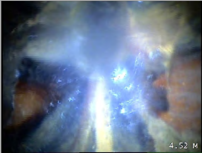
Line of drain/sewer deviates down
