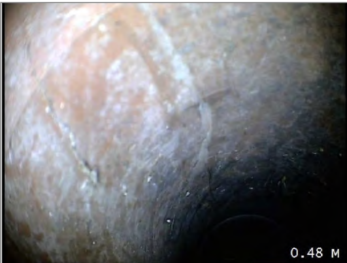
Line of drain/sewer deviates down
