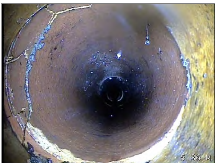
Fracture circumferential from 8 to 12 o'clock
