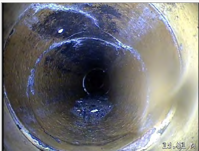
Crack circumferential from 8 to 3 o'clock
