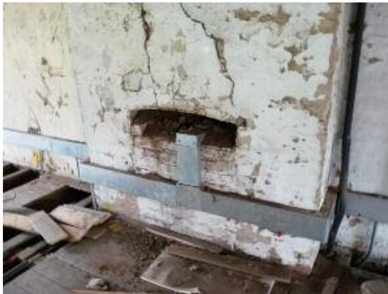
Fig.19: blocked fireplace in first floor servants' room, over central entrance block
