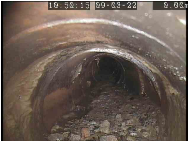
USX_96682c14-87e8-4f9c-8cd7-850dc85c04b4_20220321_151034_333.jpg, 00:00:30, 0.01 m Settled deposits, coarse, 15% cross-sectional area loss
