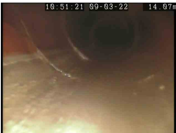
USX_d93a463c-32b1-47e3-9606-291f37a0c3ca_20220321_162520_364.jpg, 00:01:37, 14.07 m Fracture, circumferential from 5 o'clock to 9 o'clock
