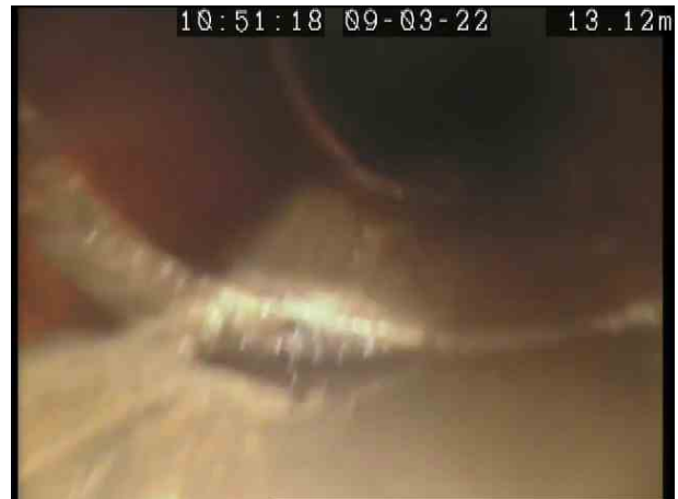
USX_3208c41a-7825-4b88-8ce2-a3c79e204f2e_20220321_162300_163.jpg, 00:01:33, 13.12 m Joint displaced, medium
