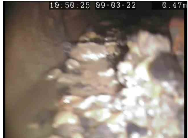
USX_3fee5d72-6eda-44c3-b356-15eea3150b77_20220321_151141_671.jpg, 00:00:30, 0.01 m Settled deposits, coarse, 15% cross-sectional area loss
