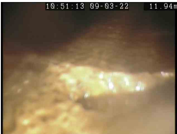
USX_ecf6a190-ef2e-4a5e-8b24-4de3b0e90d24_20220321_155113_152.jpg, 00:01:28, 11.80 m Open joint, medium
