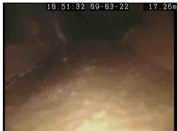
USX_4fd1bfd2-1693-4110-8f67-a645165945a3_20220321_163005_867.jpg, 00:01:47, 17.26 m Settled deposits, fine, 10% cross-sectional area loss
