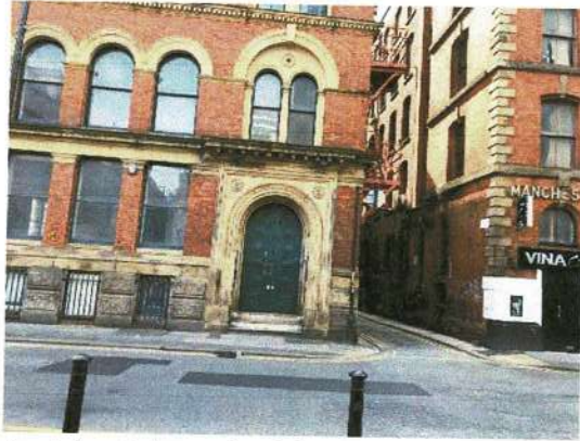
Front door to be overhauled and redecorated.
