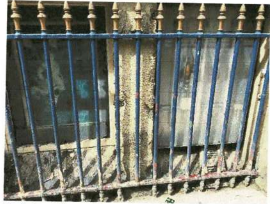
Typical cast iron railing to be redecorated and indent repairs to mullions behind.
