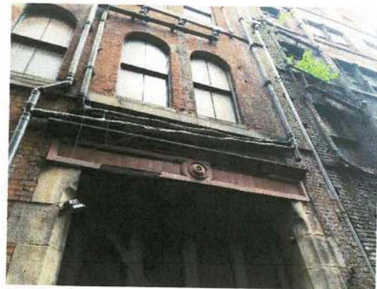
Lintel and stone jambs to Reyner Street loading bay require repair. Vegetation above to be removed.
