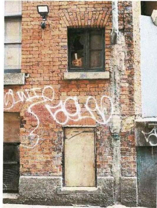
Clean off graffiti and fit new panel to redundant opening as temporary measure. Redec as windows frames.
