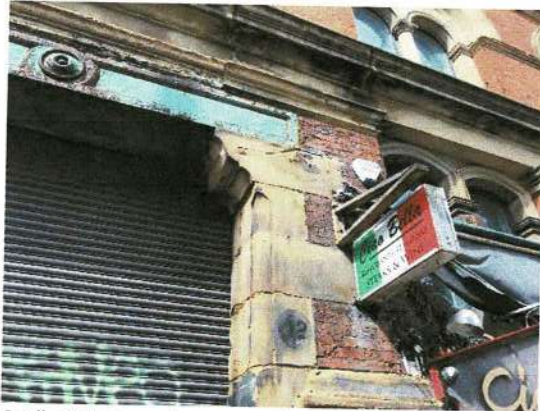
Spalled stone and masonry. (image taken prior to current works)
