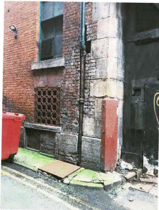
Masonry to be repointed and ventilation grille redecorated.
