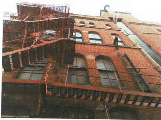
Reyner Street escape stair and ladder to be overhauled and redecorated.
