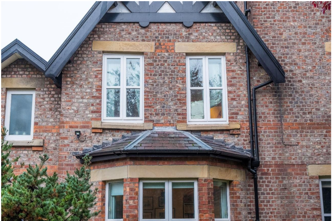
Area of work on West elevation. Defective arch obscured behind the bay window roof
