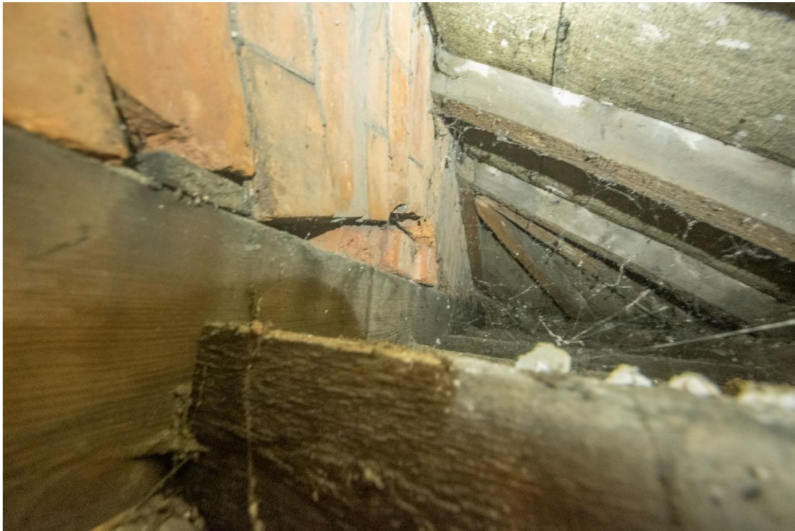
Example image of the existing, defective arch. Refer to SE's Survey Record Drawing for more.
