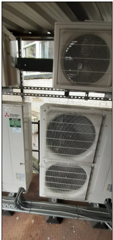
Existing Condenser Location
