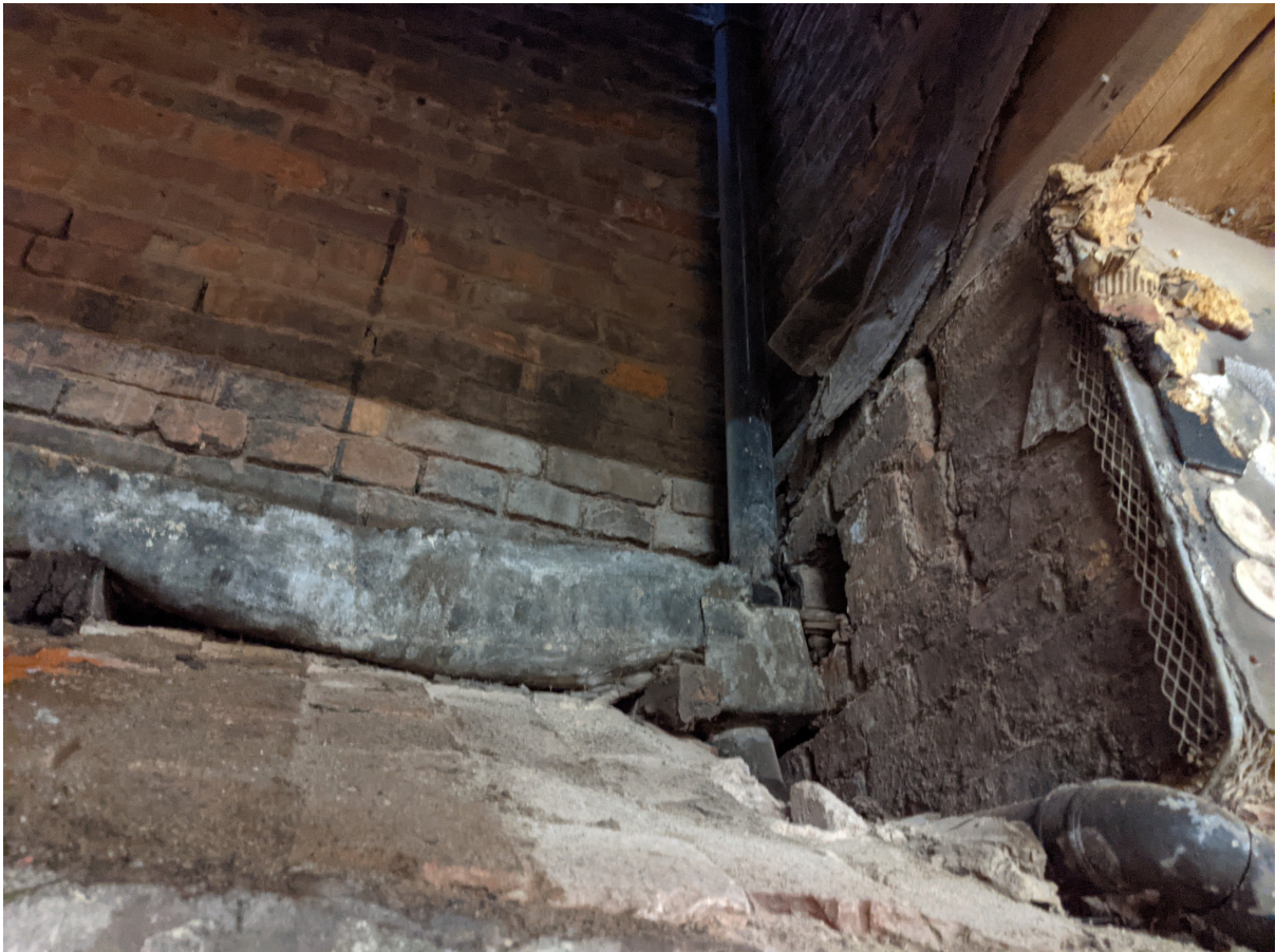
Failed lead guttering uncovered following strip-out.
