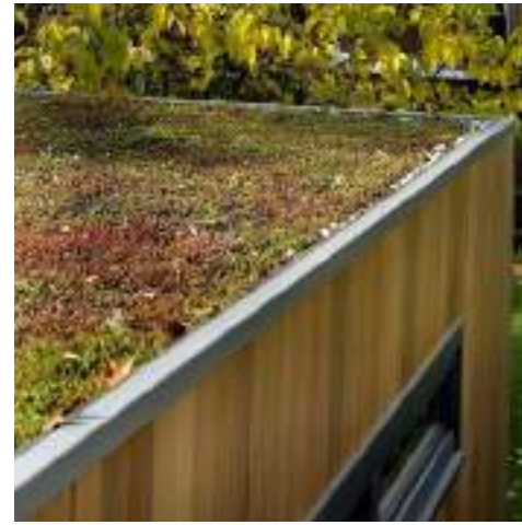
Modular sedum green roof
