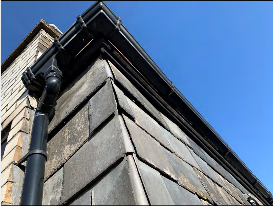
Photograph A2.5: Gaps underneath fascia board.
