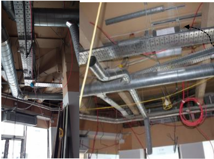
IMAGES SHOWING THE EXISTING INSTALLATION BEHIND THE PLASTERBOARD CEILING. IMAGES TAKEN DURING THE CONSTRUCTION PHASE BACK IN 2016
