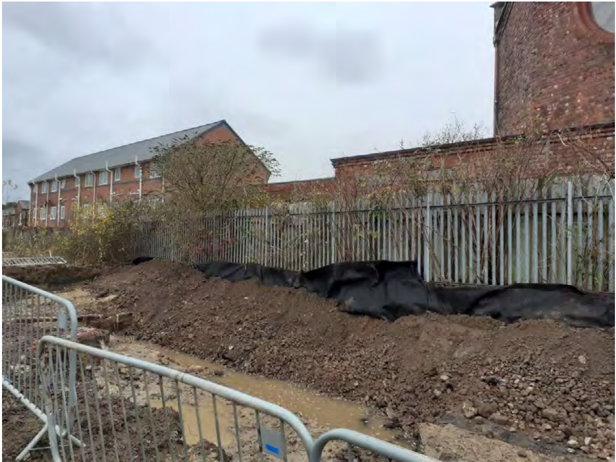
Pic 3 - JK area 1 with cutex along fence boundary
