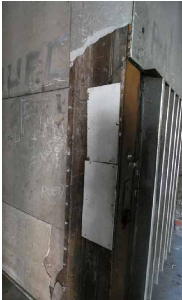
3.36 Lift shaft in G004, Ground Floor
