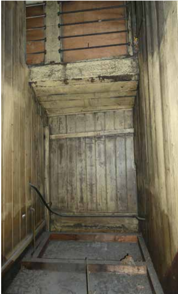
3.101 Boarded over staircase off FF010
