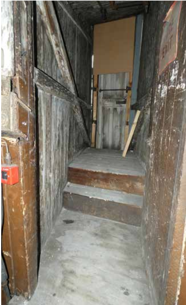
3.98 Fire escape passage, FF007
