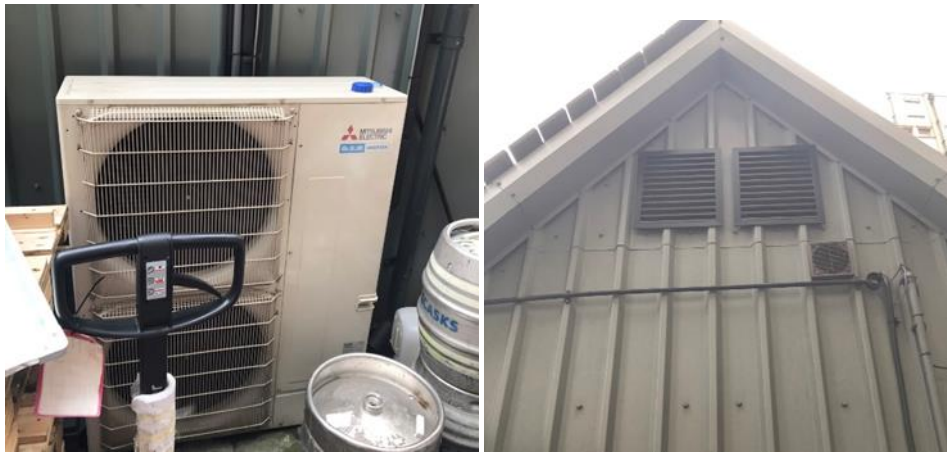
Figure 5 Photographs of currently installed items of plant (condensers – left, extract fan – right)
