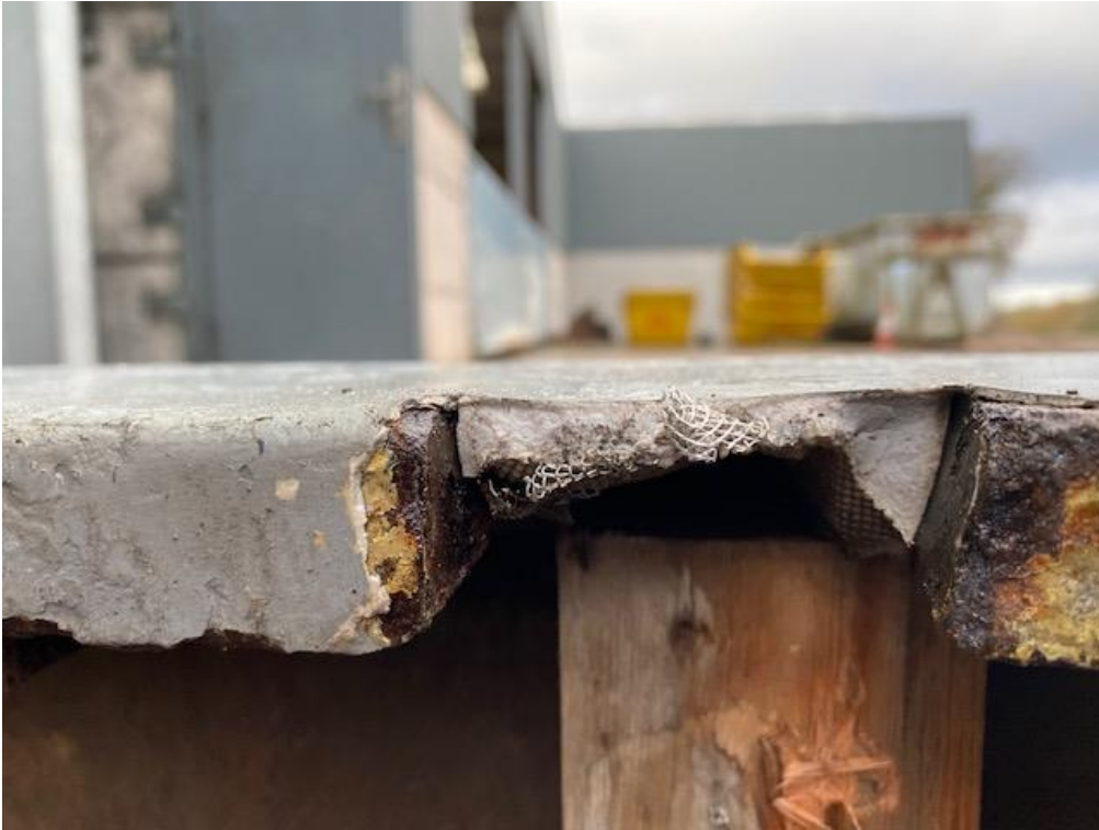
Fig.06 – Photograph of poor-quality previous repairs to cast iron column
