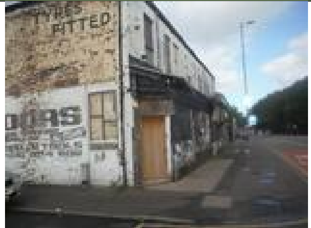
P4: Terraced properties belonging to 782 to 786 Stockport Road
