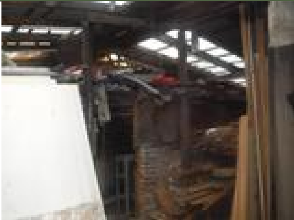
P10: Stored construction materials were present within the interior of the properties
