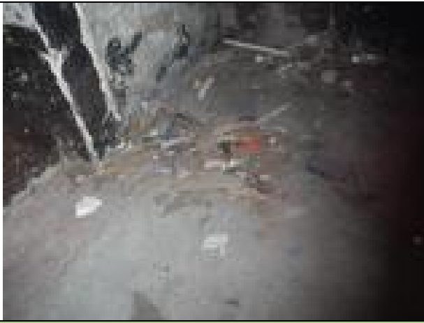
P7: The interior of the properties were generally in a poor state of repair
