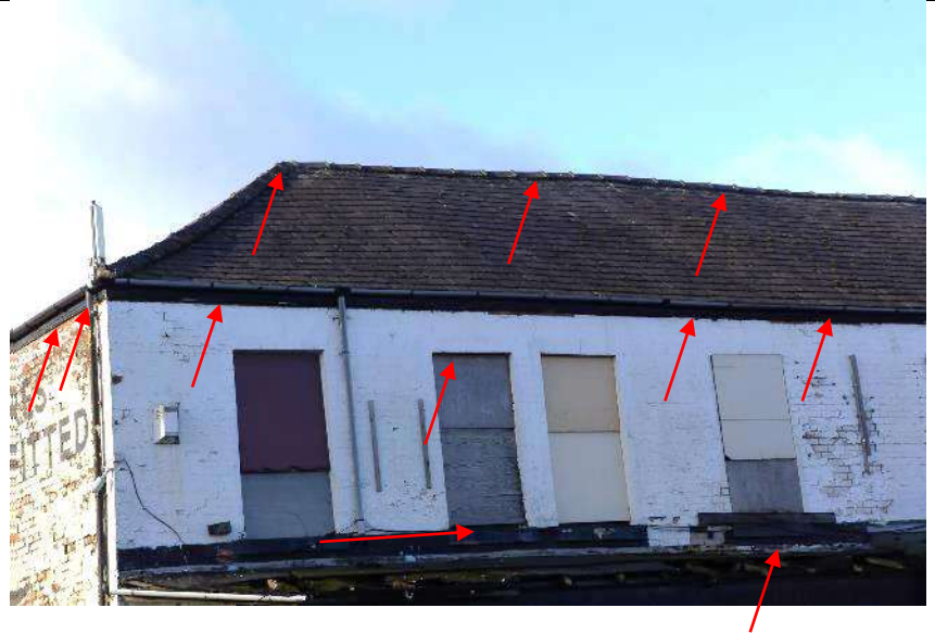
Fig.4: south and east elevation of building B1. Arrows mark the location of examples of gaps and cracks which form potential roosting features for bats, or entry to the building for birds.
