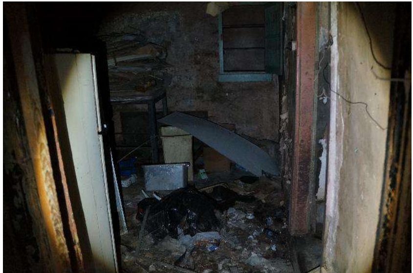
Fig.11: B1 example of inaccessible area and debris covering the floor.
