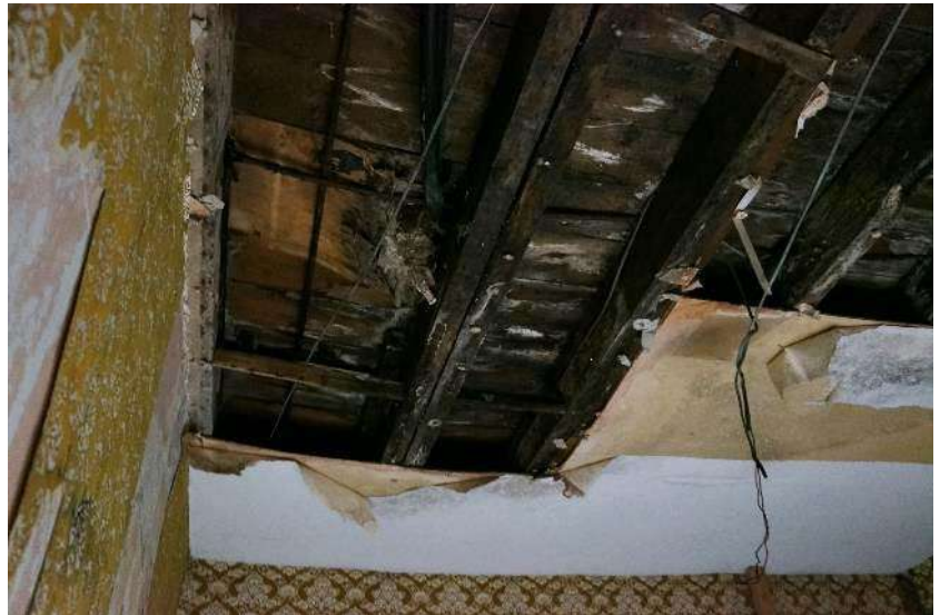
Fig.10: B1 Example of collapsed ceiling.
