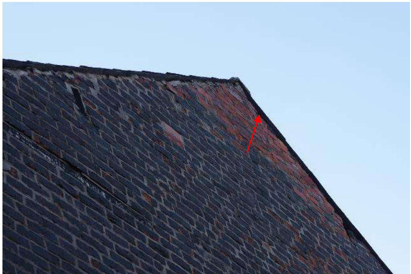
Fig.5: Close up of the north gable end of the B1 with gaps in the mortar at the apex
