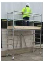
Low-level Access tower <2.5metres
