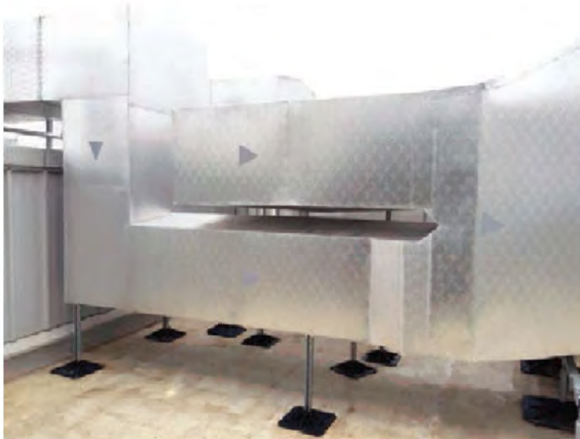
Typical duct installation
