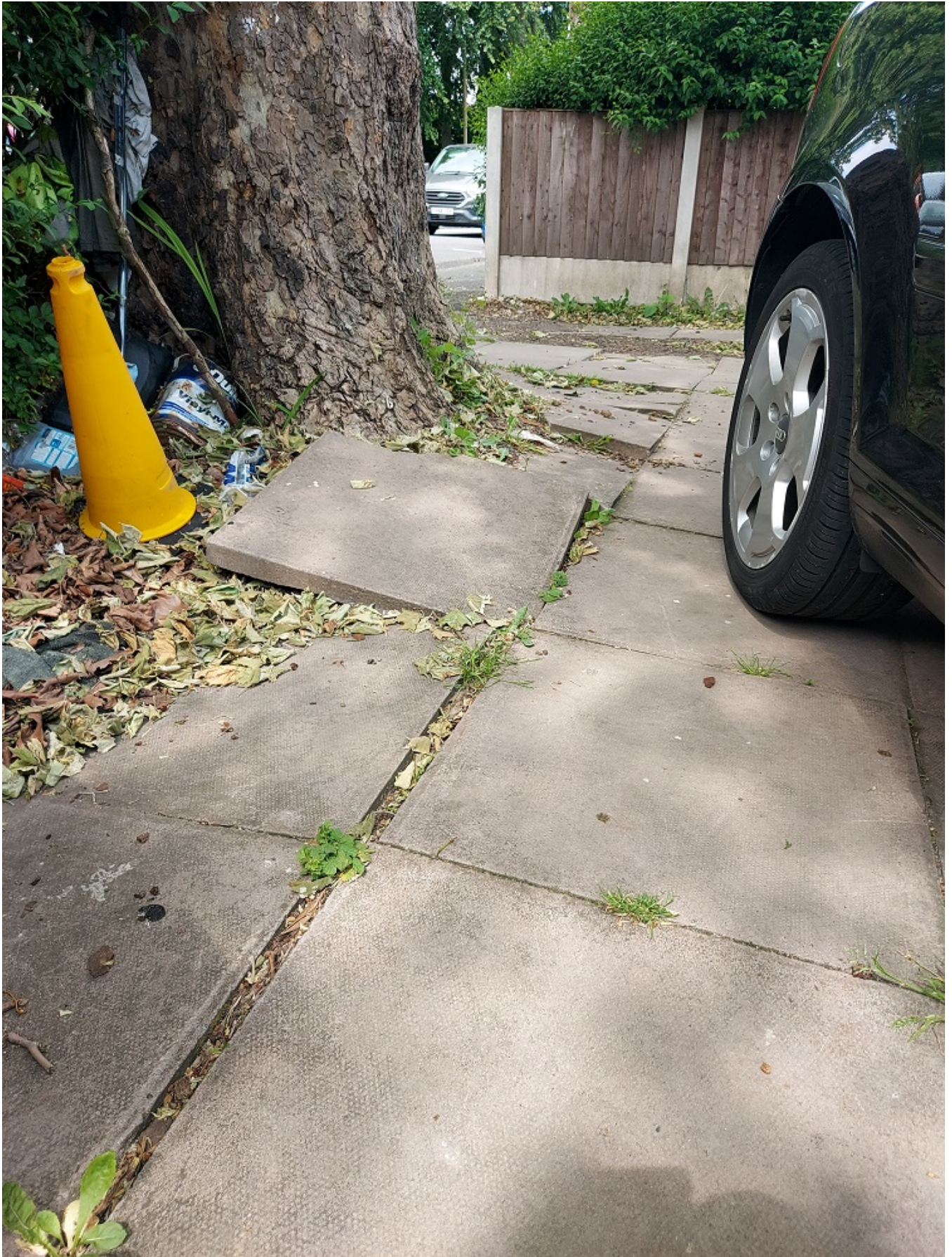
Figure 2 Roots from T1 are disrupting the driveway of 621 Burnage Lane
