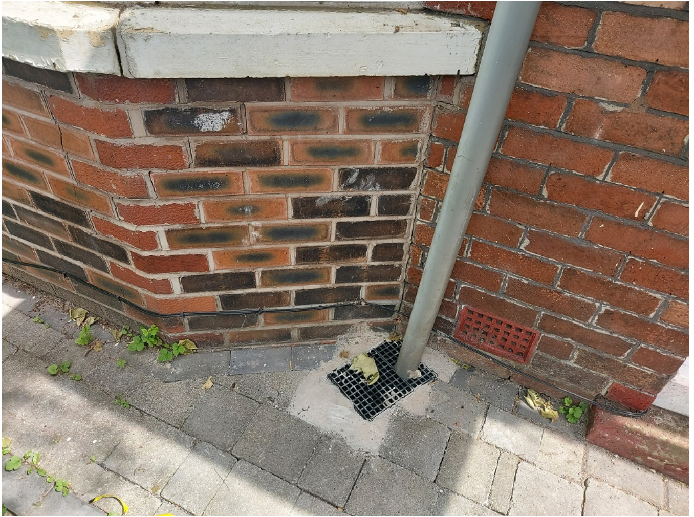
Figure 1 Cracking is evident in the brickwork of the bay windows
