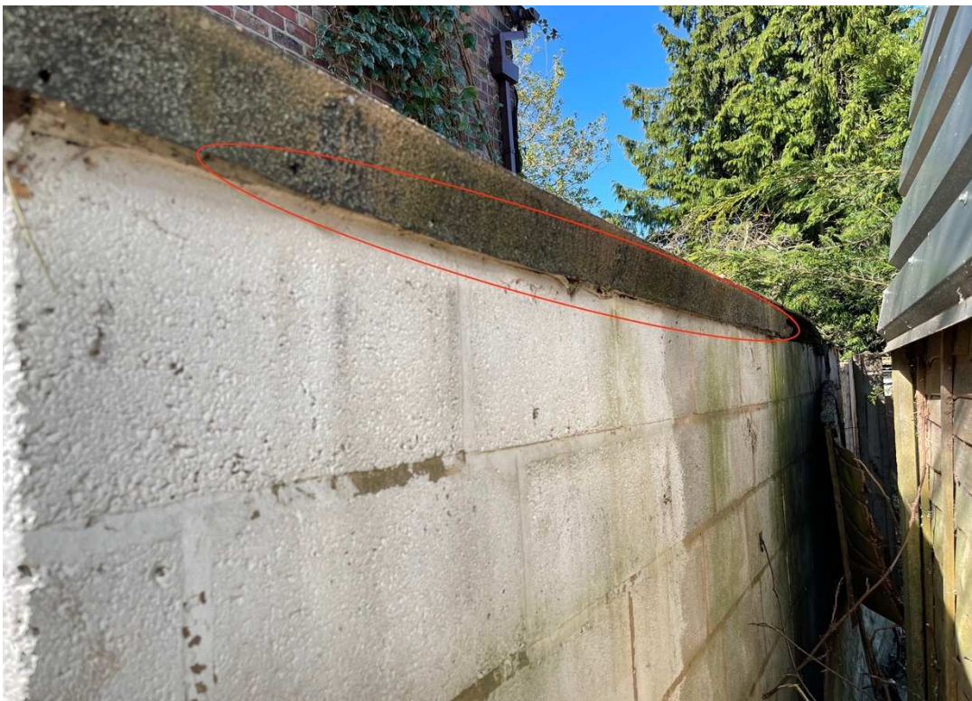
Plate 4: Overhanging felt and damage to wooden fascia behind forms gaps
