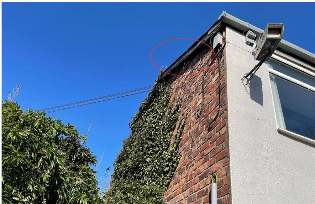
Plate 2: wooden fascia on southern aspect gable end forms small cavities where it is fixed to the wall
