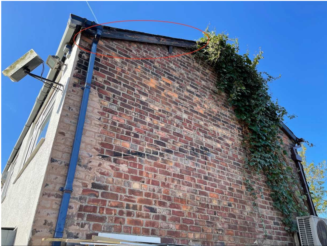
Plate 3: wooden fascia on southern aspect gable end forms small cavities where it is fixed to the wall.
