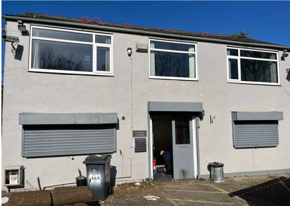
Plate 1: Missing mortar on ridge tiles at various locations
