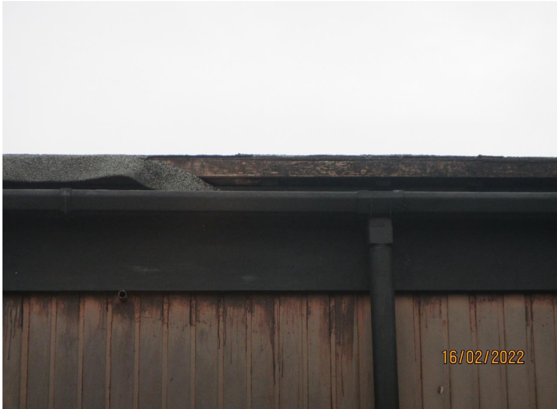
Photograph 6 – The north-eastern aspect of the hipped extension where the bitumen roof felt and the timber fascia have degraded, creating a gap into the structure.
