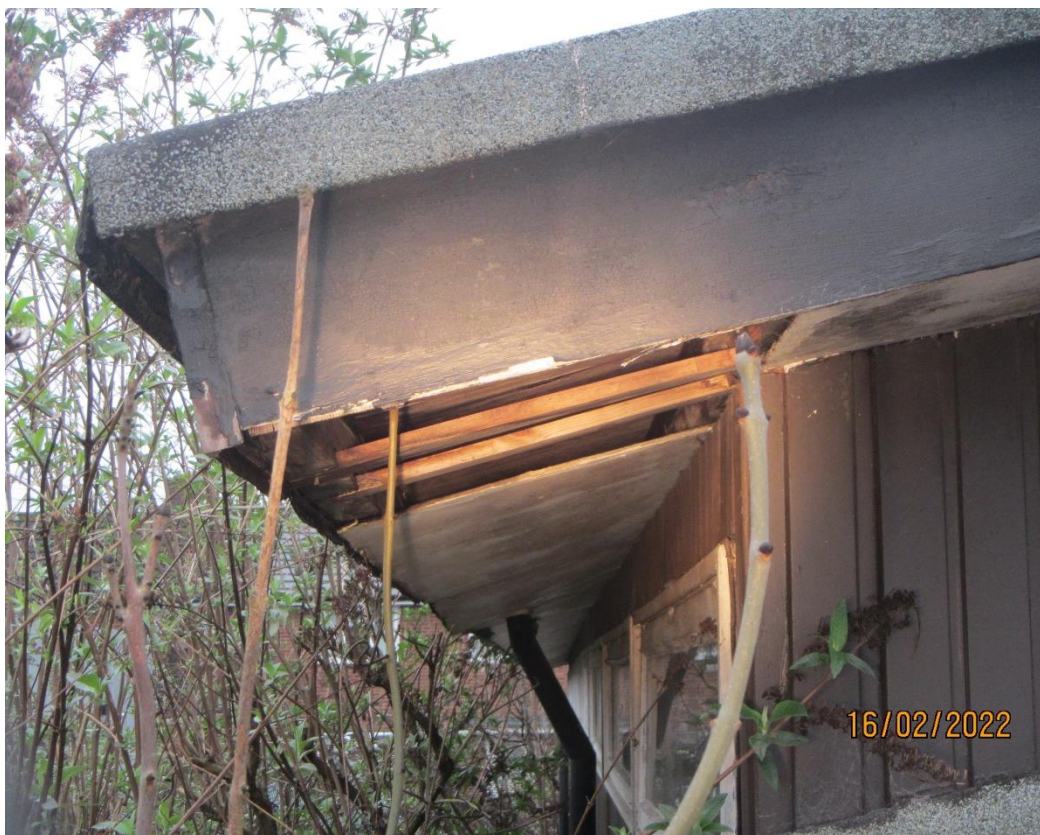
Photograph 4 – Damaged timber box soffits creates a generally unsuitable feature for roosting bats due to the absence of internal roosting features, and cluttered access point.
