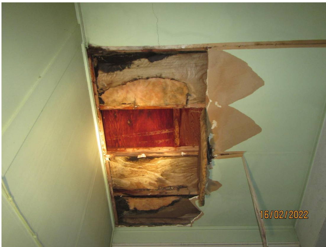
Photograph 9 – The water damaged roof at the north-eastern end of the main hall, revealing the single skin plywood, timber beam and insulation construction of the roof.
