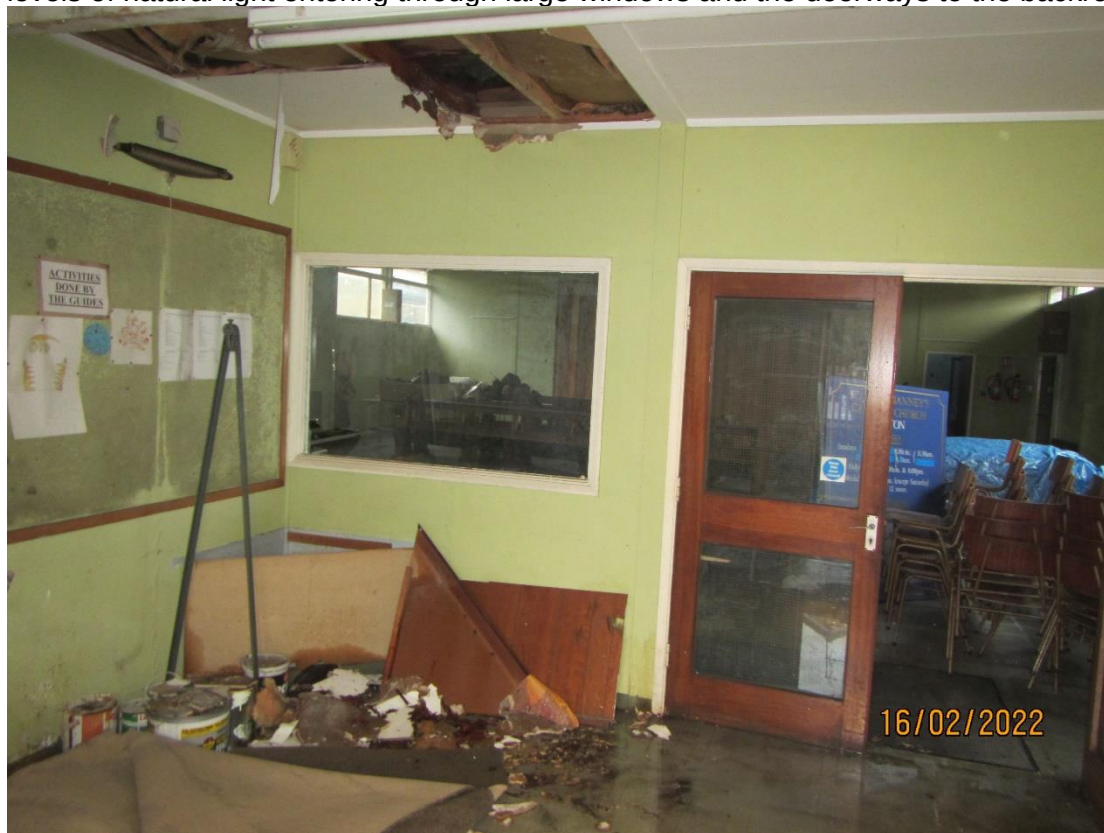
Photograph 12 – A large hole in the single skim plywood ceiling of the foyer leading to the hipped extensions loft void, which has been created through water damage.
