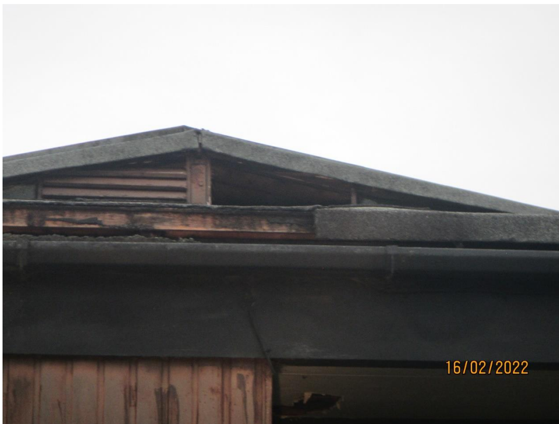
Photograph 7 – A close up of the damaged timber ventilation feature which faces north-west on the hipped roof extension and provides easy access into the structure.
