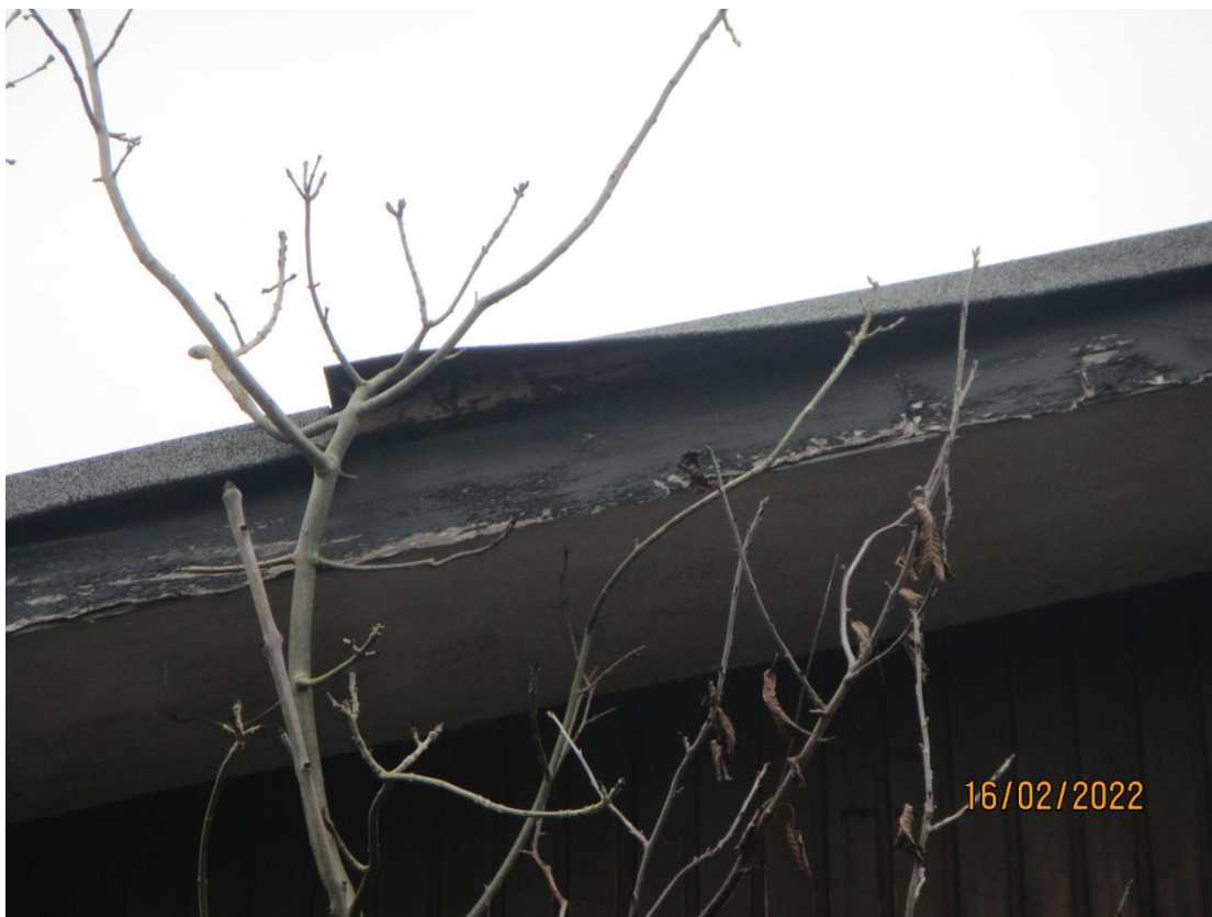
Photograph 2 – The south-western aspect where a section of the bitumen roofing felt has raised from the pitched roof. Access under the felt is impeded by the raised timber batten.
