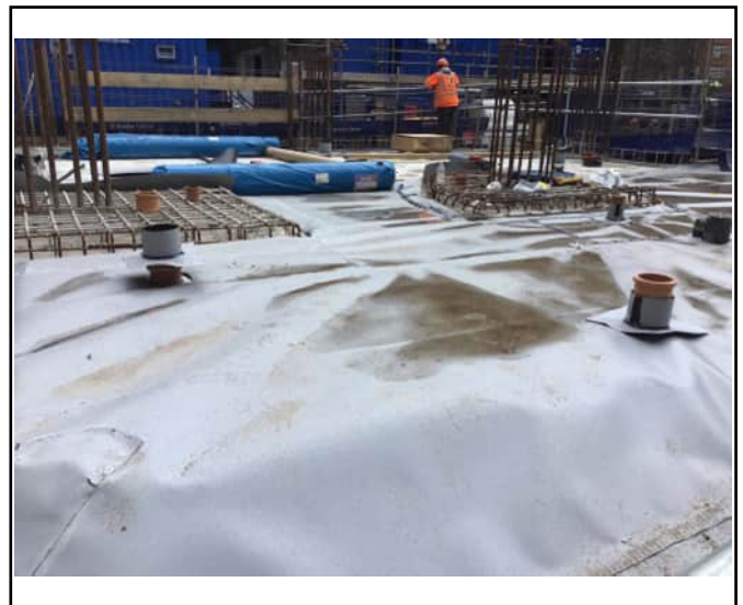
Overview of verified installation
