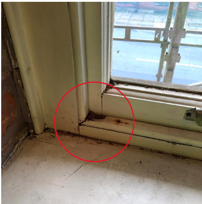
Figure 10. (left) Photographs existing sash window, part of existing staff bead is in poor condition, showing decayed timber beading.
