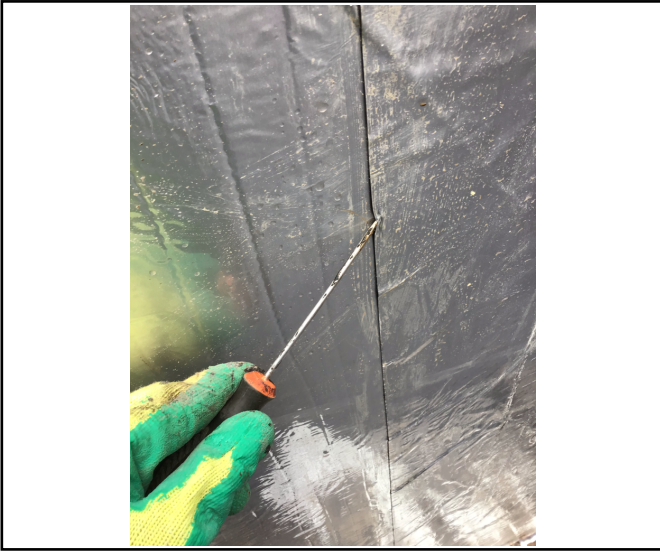
Pick and probe test carried out to D7
