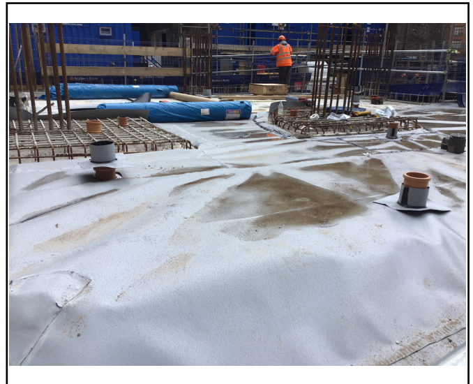
Overview of verified installation
