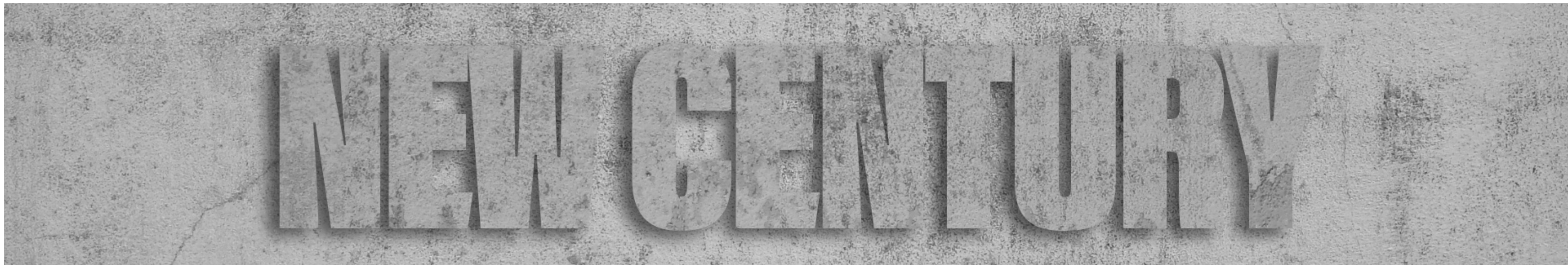
CONCRETE LETTERS FIXED TO ORIGINAL EXTERNAL CONCRETE WALL APPROX SIZE 3000 X 500 X 15MM
