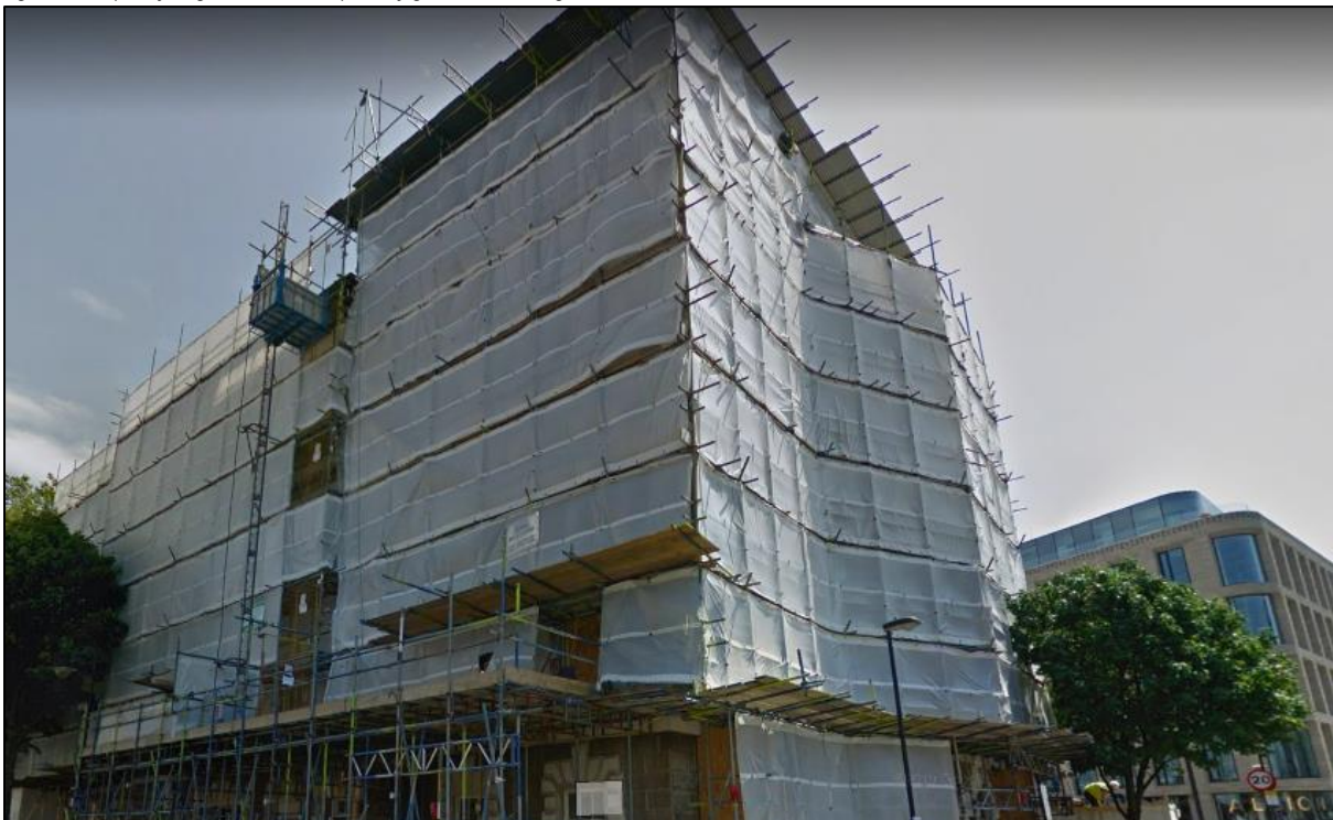
Fig. 2: Example of negative visual impact of generic sheeting - 2016
