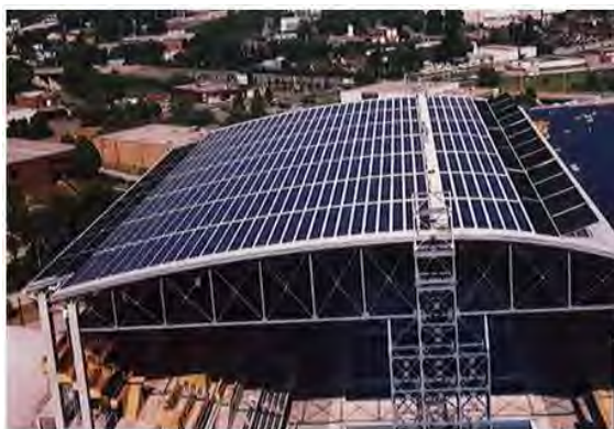
Image 14 - Solar Photovoltaics (PV)
