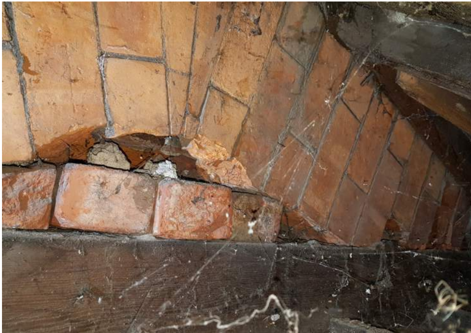
Figure 5: Crudely formed relieving arch spreading on abutments owing to broken brick and timber packers to awkwardly tapering joint either side (see Fig. 6)
