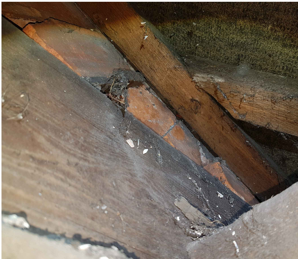
IMAGE 03: VIEW OF RIGHT-HAND BEARING (AS VIEWED EXTERNALLY. SEE IMAGE 01) SHOWING TIMBER WEDGES AND CUT BRICK PACKERS TO AWKWARD TAPERED END OF RELIEVING ARCH. NOTE LOOSE CHARACTER OF CUT BRICK UNITS AS ARCH SLIDES ALONG BEAM.
