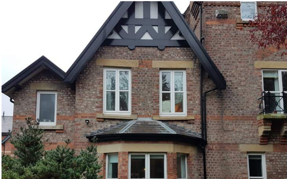
Figure 1: G.A. view on W gable showing position of projecting bay window and area of structural activity overhead.
