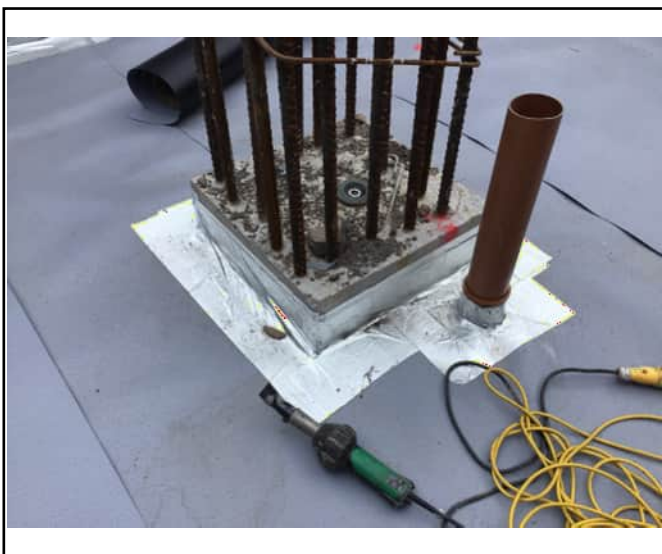
Penetrations in Gridlines 11/6:E/G
