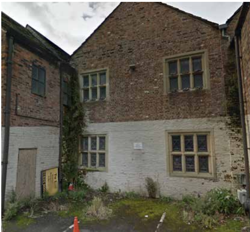
Figure 17- rear extension showing build-up of vegetation and poor drainage (Google Street View, 2014).
