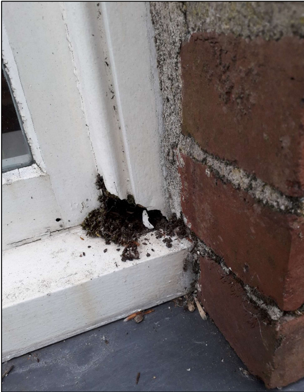
Figure 7: View of Rot to Window.
