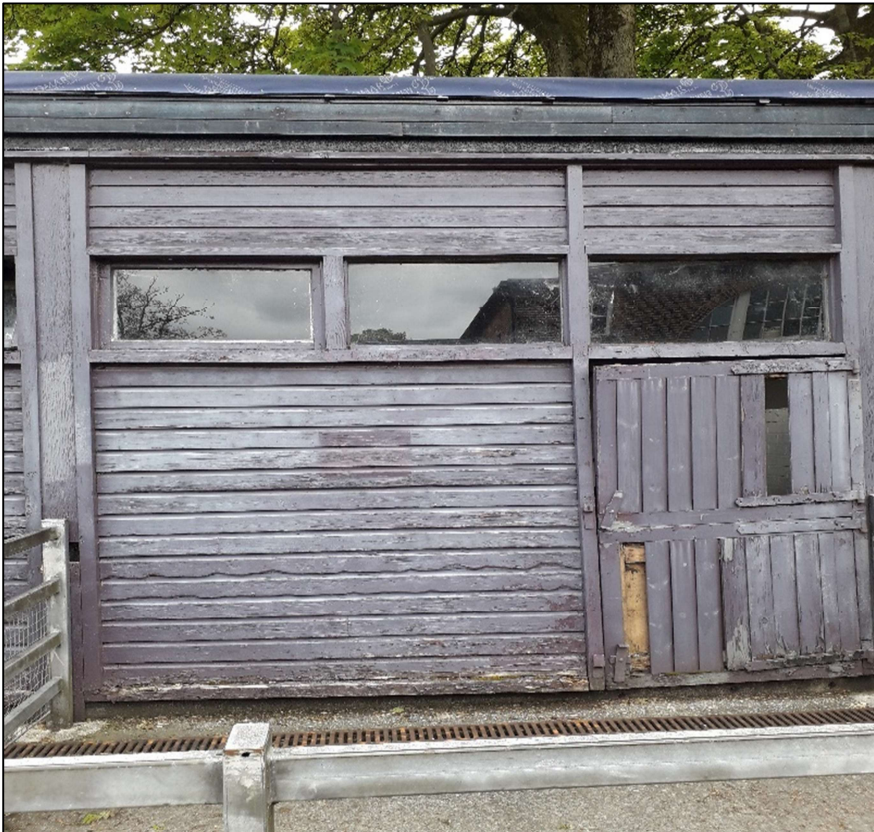
Figure 5: View of Rotted / Missing Boarding to Stable Block in Courtyard Area.
