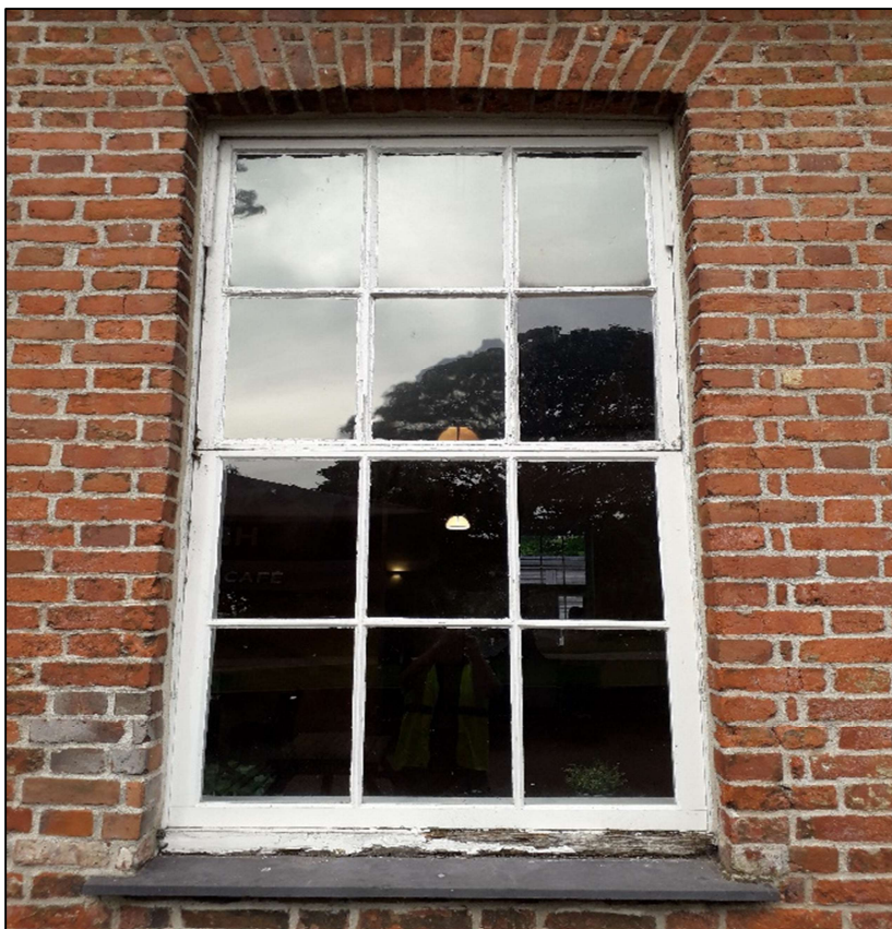
Figure 6: View of Rotted Timberwork to Cill of Vertically Sliding Sash Window.
