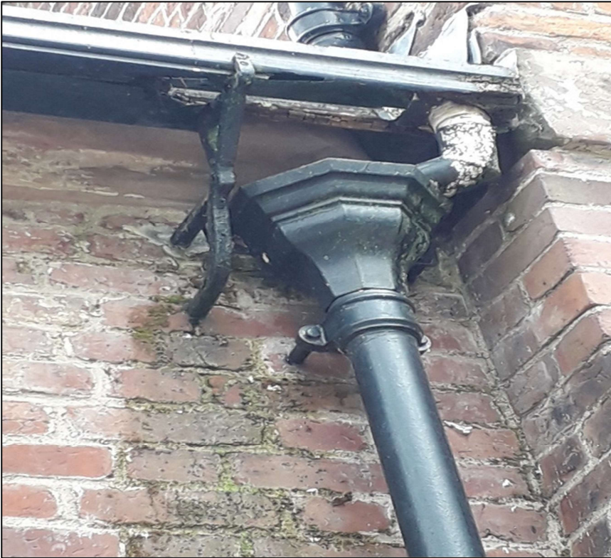
Figure 3: View of Existing Timber Guttering. Completely Rotted Through & Leaking.
