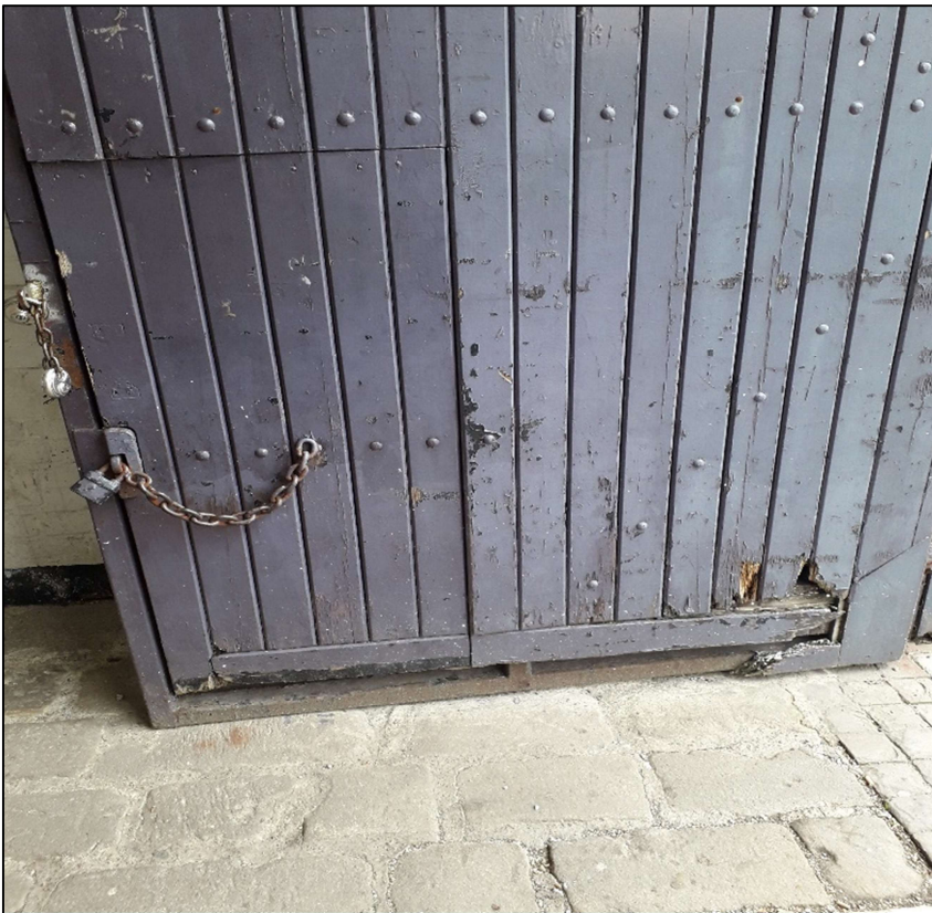
Figure 4: View of Rotted / Missing Boarding to Courtyard Entrance Doors.
