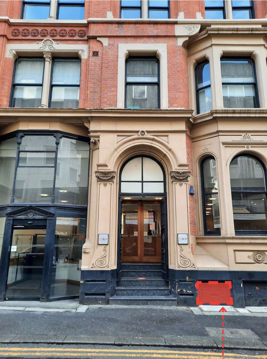
Dry Riser Inlet
