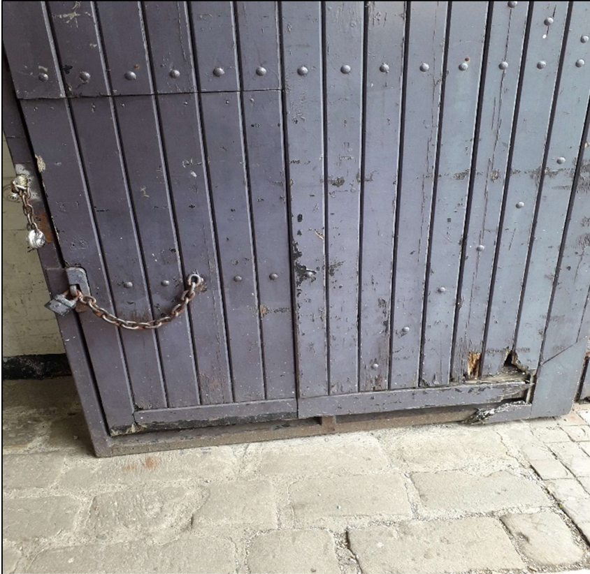
Figure 7: View of Rotted / Missing Boarding to Courtyard Entrance Doors.
