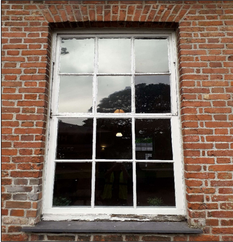
Figure 9: View of Rotted Timberwork to Cill of Vertically Sliding Sash Window.
