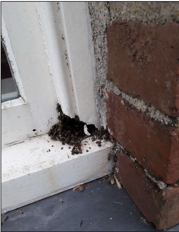
Figure 10: View of Rot to Window.
