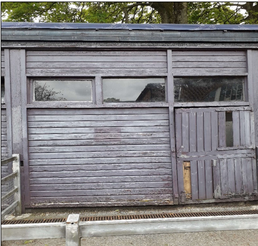
Figure 8: View of Rotted / Missing Boarding to Stable Block in Courtyard Area.
