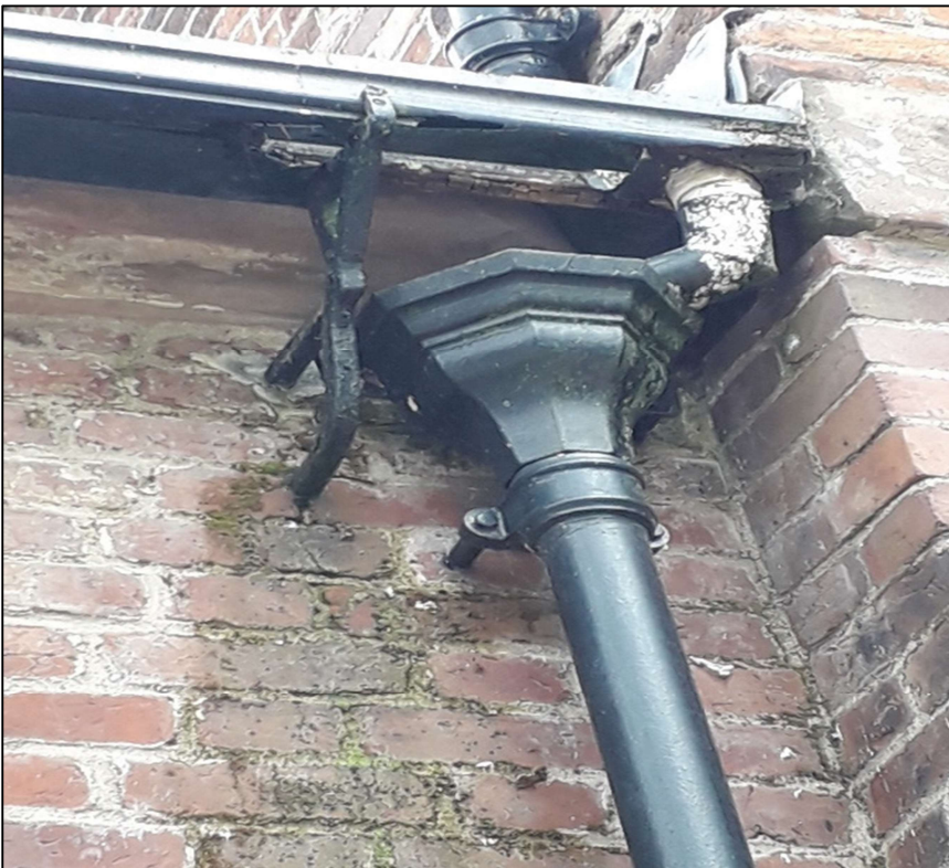
Figure 6: View of Existing Timber Guttering. Completely Rotted Through & Leaking.
