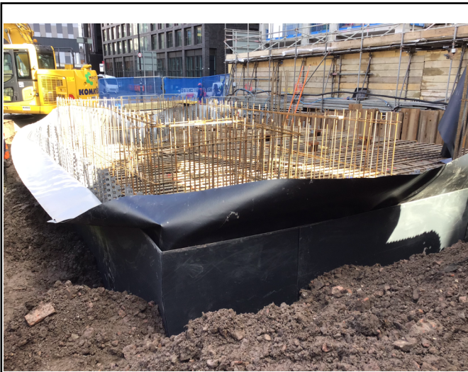
Protection board to base of crane
