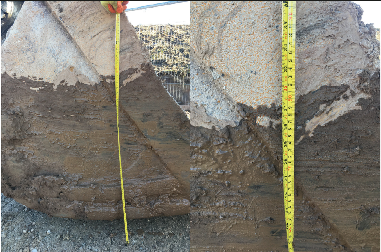
Plate No. 2: Depth of infilled material
