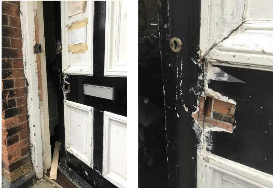
Damage to timber panelled doors and frames
