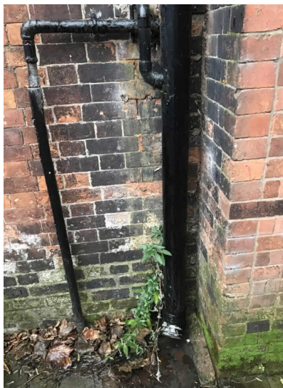
Damage to low level brick
