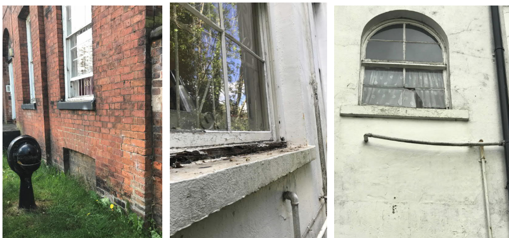
windows in various states of disrepair with security bars to vulnerable ground floor
