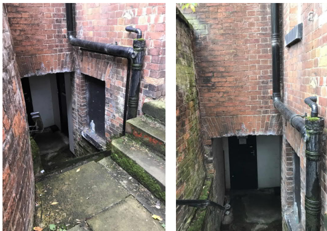
Leaking downpipes and stacks
