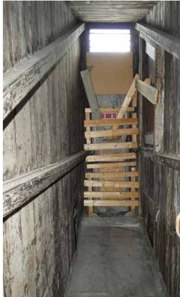
3.102 Fire escape passage, FF011
