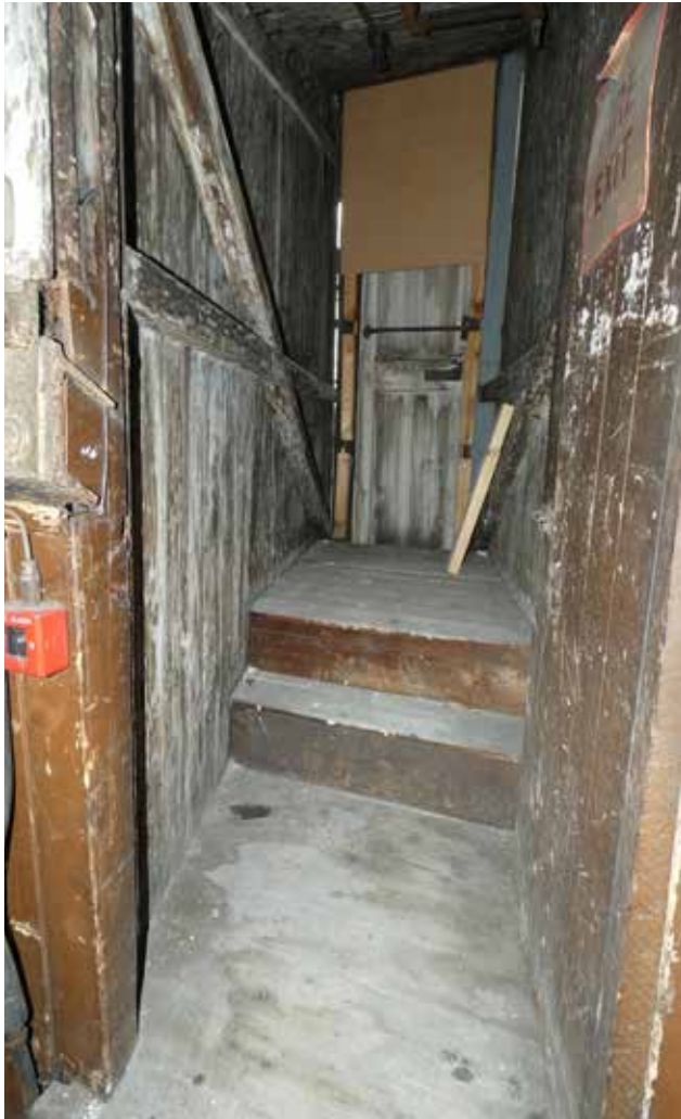
3.98 Fire escape passage, FF007
