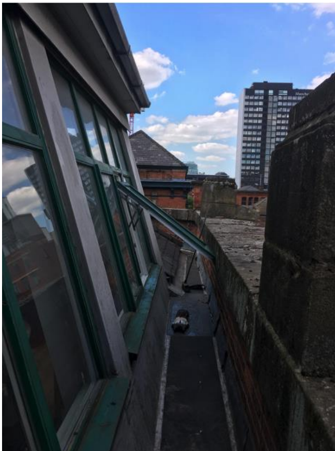
(Figure 10 Parapet gutter showing damaged caused by water to the wooden windows and gutter)
